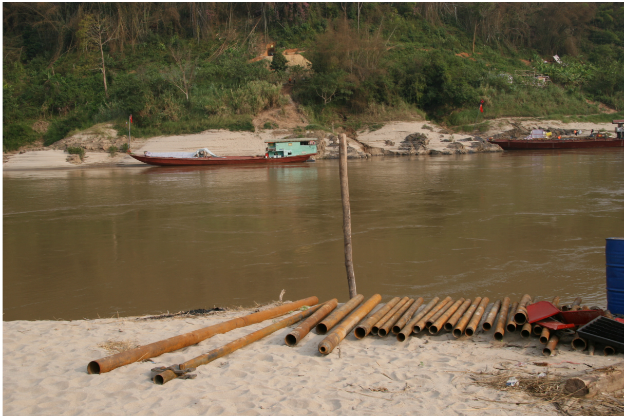
Surveying and drilling work at the proposed site of the 1,320 MW Pak Lay dam on the Mekong mainstream, northern Laos. In June 2007, the Lao government signed an MoU with Sinohydro and China National Electronics Import and Export Corporation to undertake a feasibility study of the dam.
