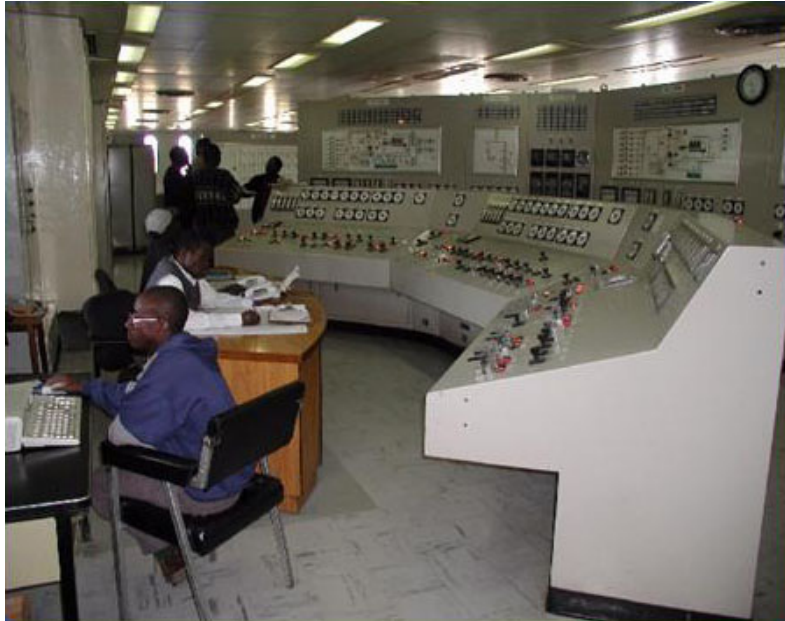
Figure 4: Olkaria I Geothermal Plant Control room Source: NAPE files
