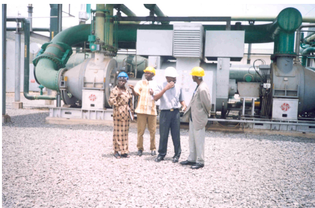
Figure 7. Mr. Mabwa Ernest (third left - white helmet) of OrPower IV explains to NAPE staff how a binary geothermal power plant works. The plant is a good example of sustainable and environmentally friendly geothermal technologies.
